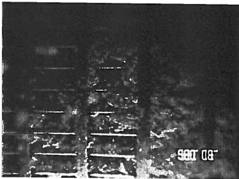
Figure 2 - Scale Formation on a Well Screen. Photo: Gary Hix. Source Arizona Cooperative Extension.
